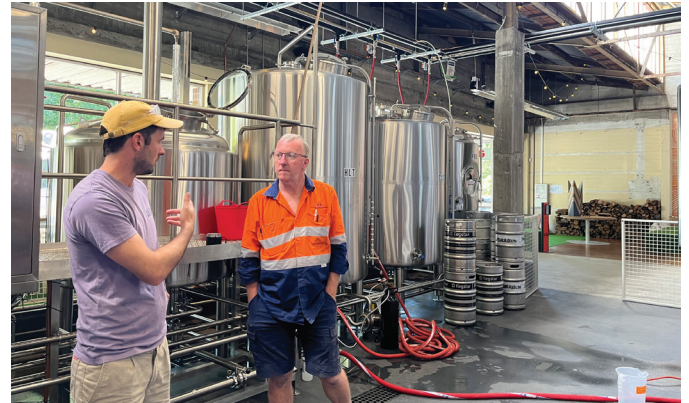
Engineering, design, supply and install of COOL-FIT was all kept in-house by Mitchell Engineering with support from GF Piping Systems Australia and Actrol Launceston
